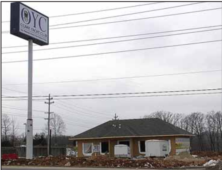
Both state and city officials agreed, the Lake area should expect to soon see an improvement in the employment picture. Construction of Ozark Yacht Club's new showroom on Bagnell Dam Boulevard is a sign of good things to come. Nancy Hogland photo.
